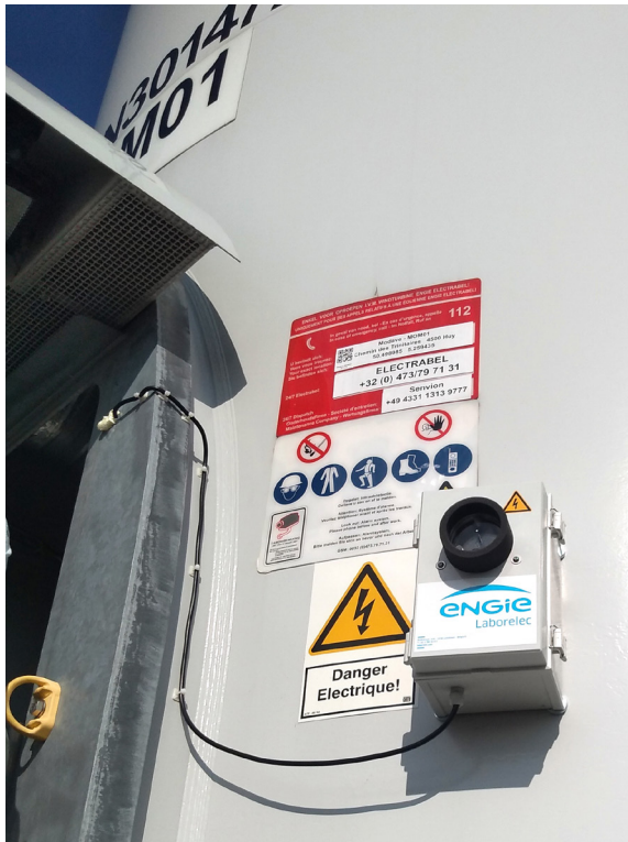
The ultrasonic detector at the turbine base
