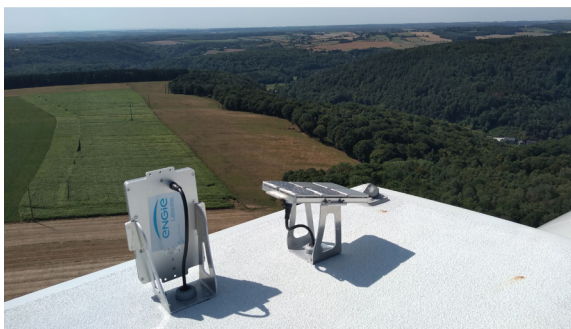
NRG deterrent speakers fixed to nacelle
