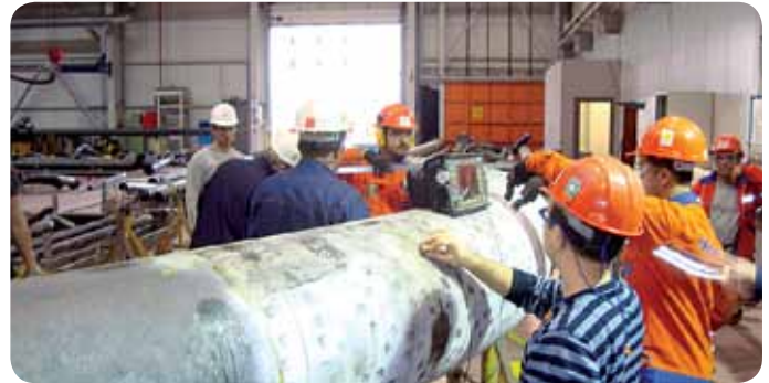
Laborelec verified manufacturing procedures to assure long-term integrity and availability of the piping.
