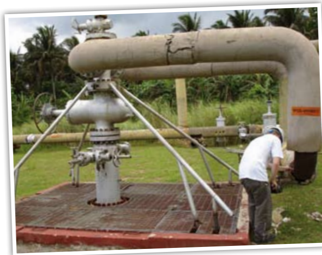
Onsite spot checks are carried out on power components.
