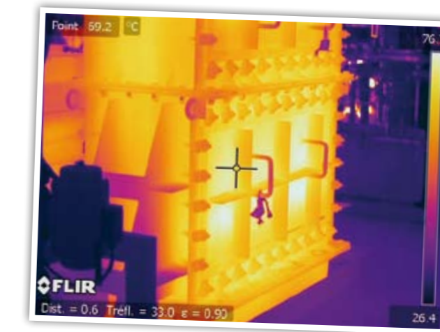
Laborelec has used infrared thermography at the Ruien power plant to locate erosion in very small areas.
