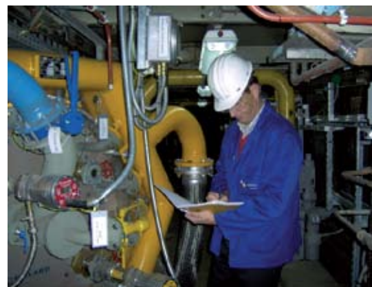
Laborelec helped the Awirs 5 gas-fired power plant with the purchase and commissioning of new low NO x burners.
