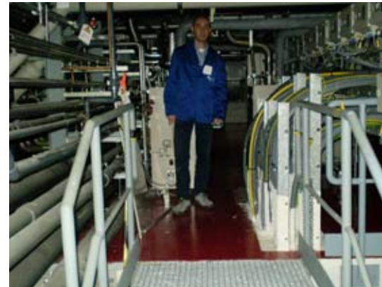
The electro-magnetic interferences with the gas detection alarms were solved by improving the grounding network
