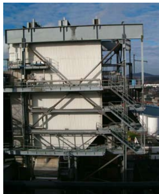
Nowadays deNO x installations are equipped with Selective Catalytic Reactors (SCR) in order to comply with the new Large Combustion Plant (LCP) directive.
