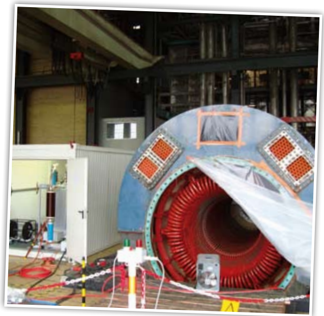
The Laborelec power sources not only identify ageing mechanisms, they also allow for trending and comparison with other generators.
